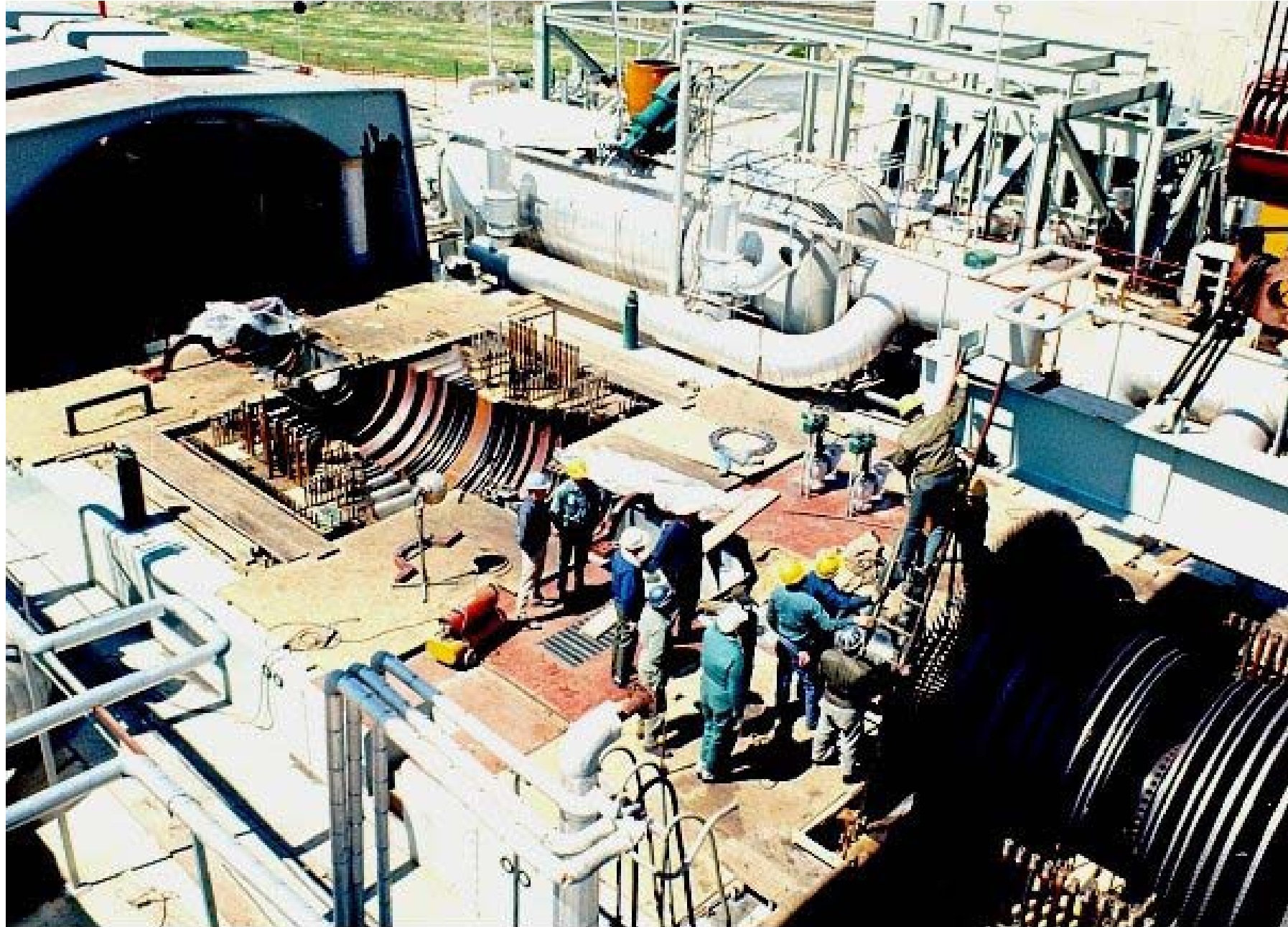
Turbine bed for a steam power station. (Courtesy of Carolina Power and Light Company)
