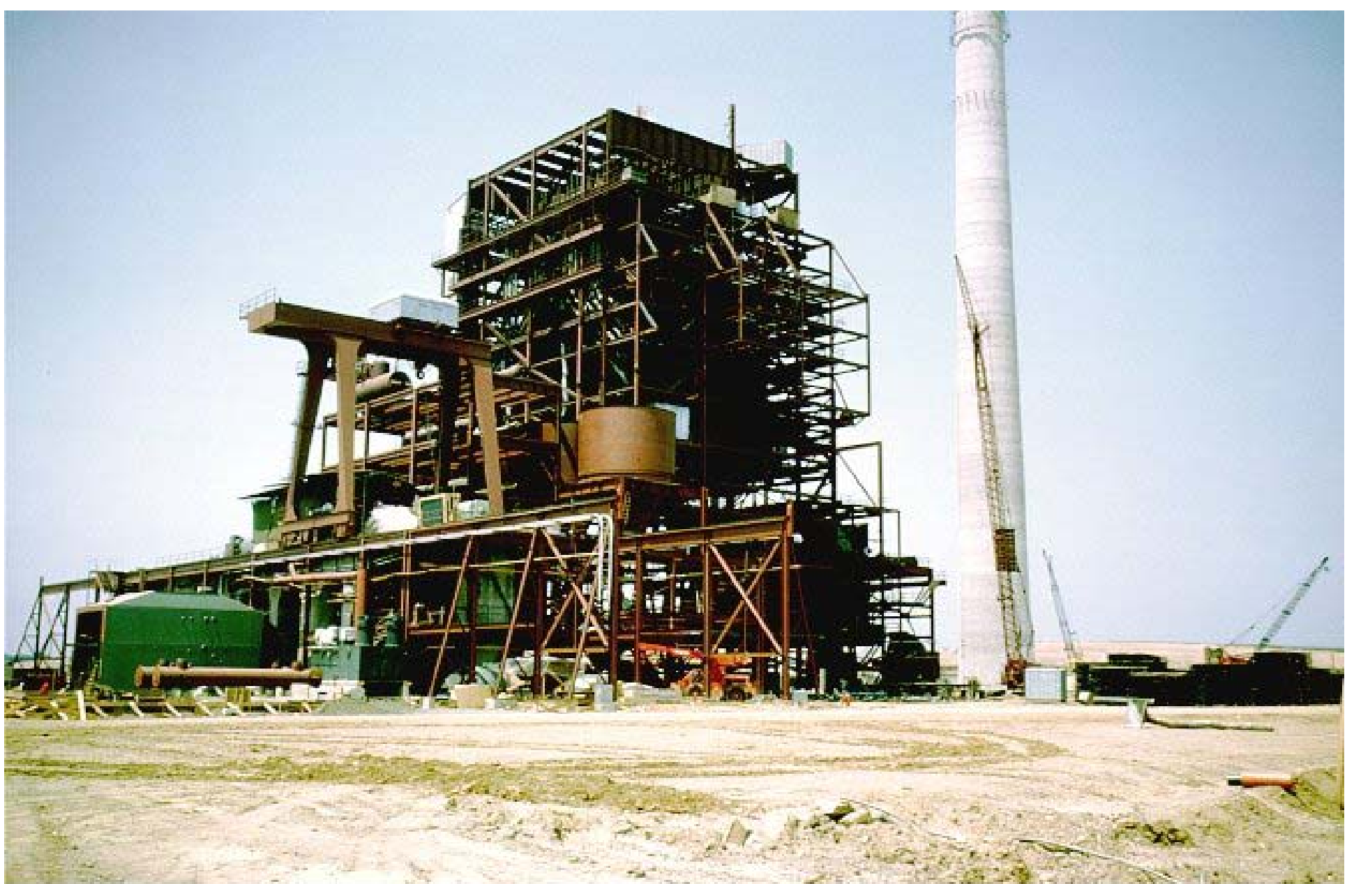
Steel structure of a steam generator at a coal fired steam power plant. (Courtesy of Carolina Power and Light Company)
