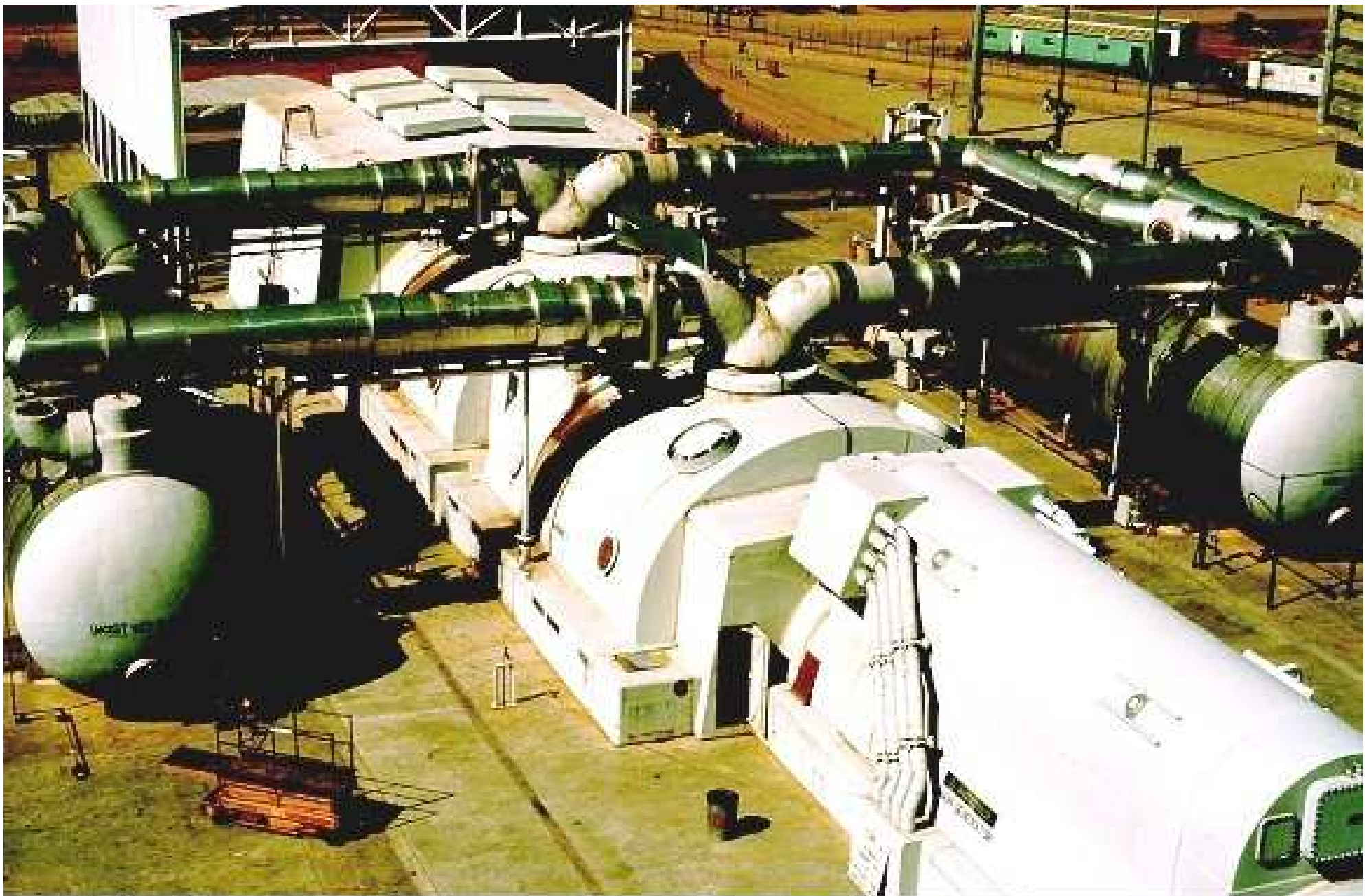
Overview of a steam turbine and main generator for a nuclear steam power station. (Courtesy of Carolina Power and Light Company)
